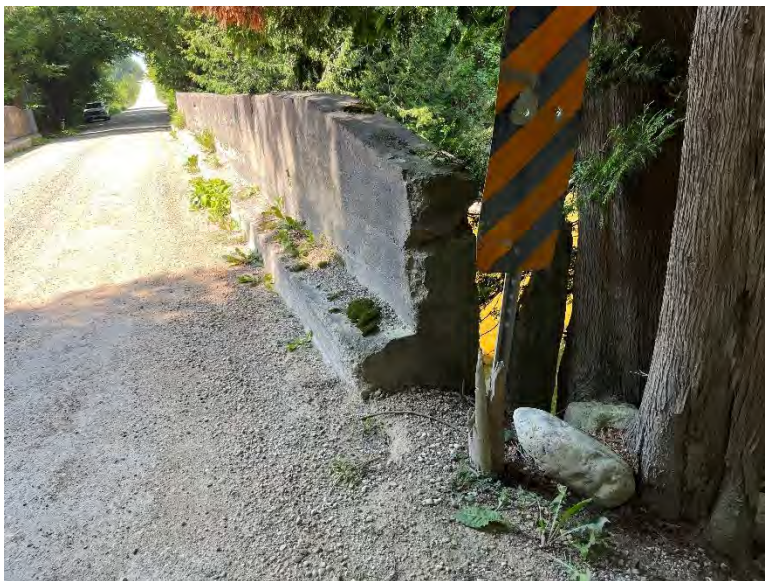
Plate 5: Detail view of gravel deck and concrete curbs and barrier. Note significant visible deterioration to concrete (A.S.I., 2023).
