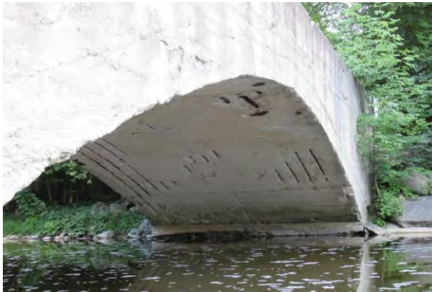
View of Exterior and Interior Soffit with Spalling and Exposed Rebar
