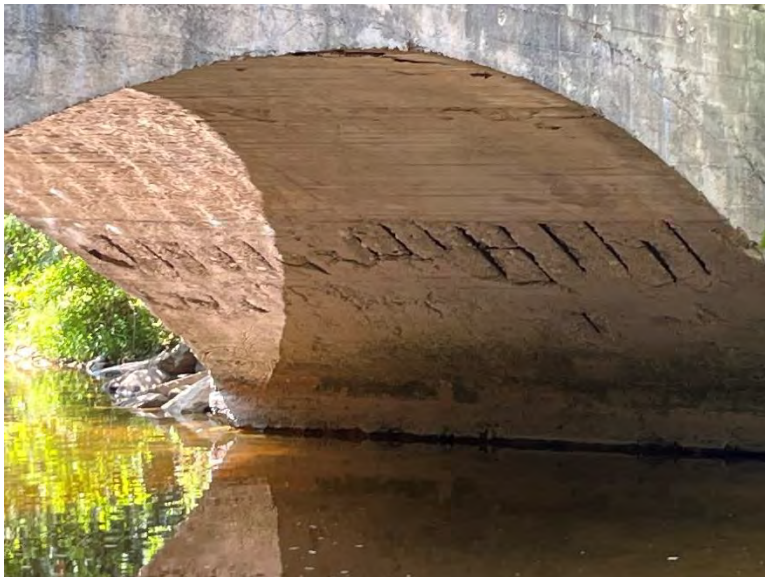
Plate 7: Detail view of barrel underside showing concrete deterioration and exposed rebar (A.S.I., 2023).
