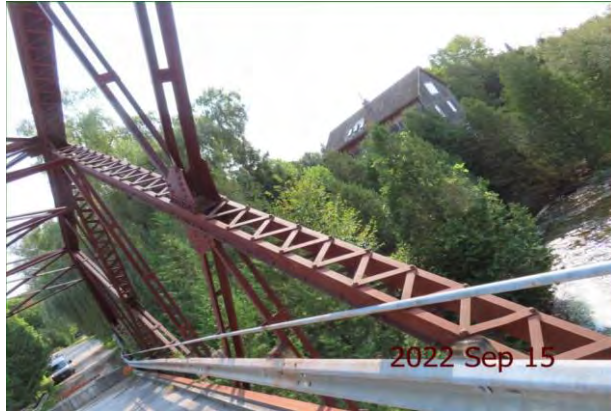
Corrosion and Impact Damage to Diagonals
