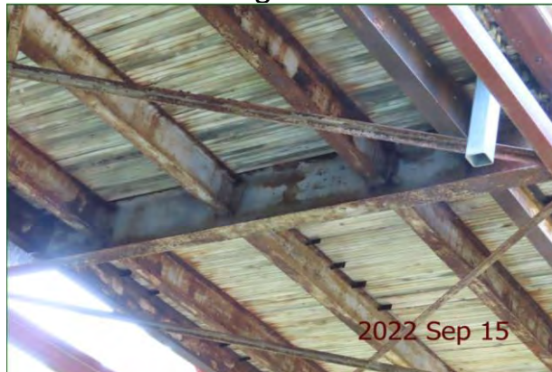
Severe Corrosion at Ends on Floor Beam
