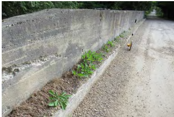
Delamination Along Parapet Wall and Vegetation and Debris on Curb
