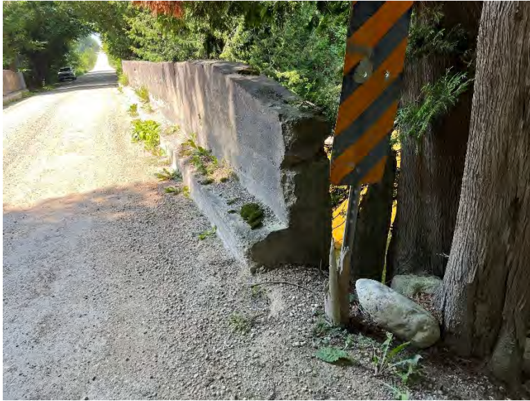
Figure 13: Detail view of gravel deck and concrete curbs and barrier. Note significant visible deterioration to concrete (A.S.I., 2023).
