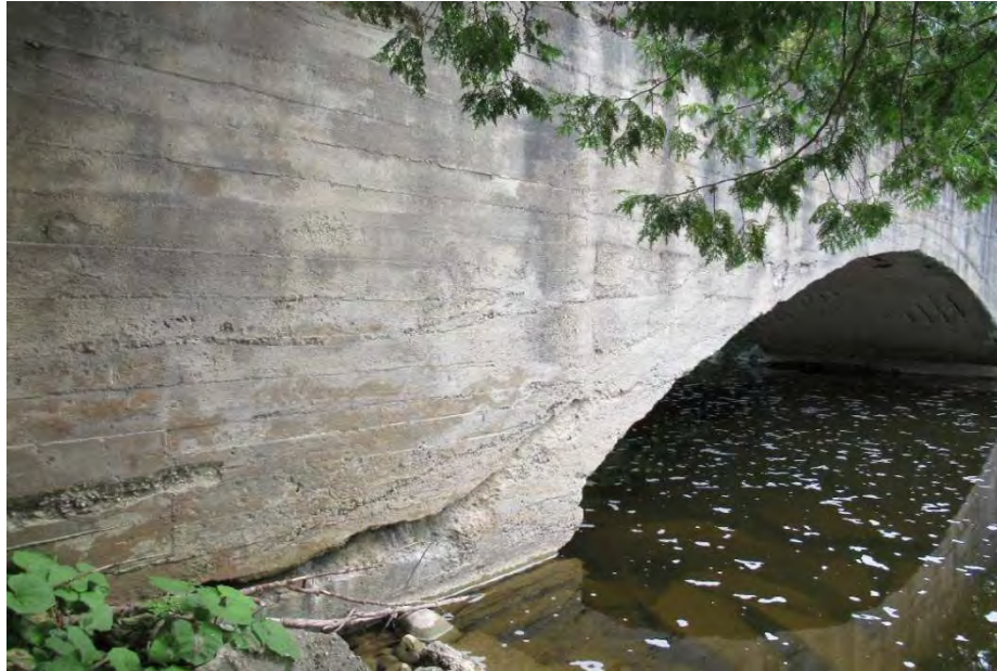
Figure 2.7 Scouring of Wingwall
