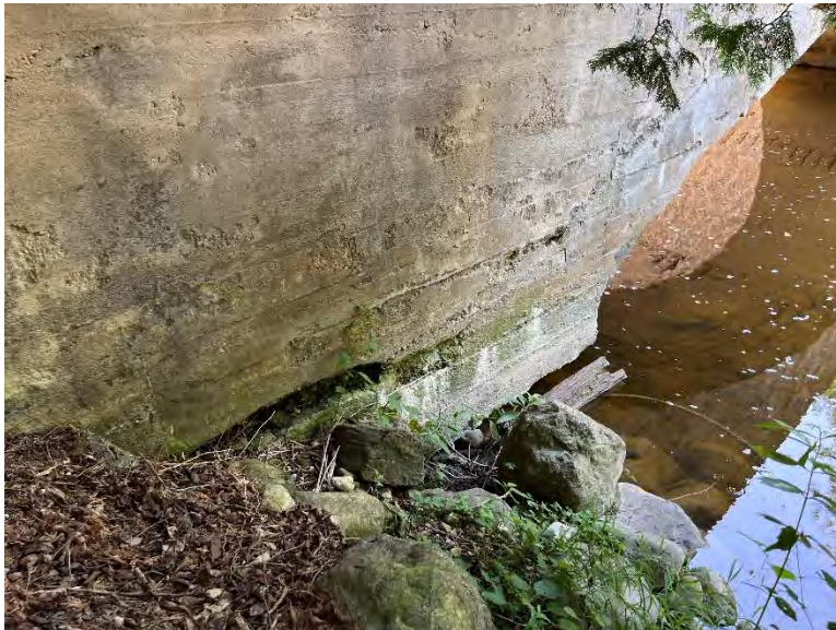
Figure 14: Detail view of north side of eastern abutment. Significant deterioration is visible at the waterline and at the berm (A.S.I., 2023).
