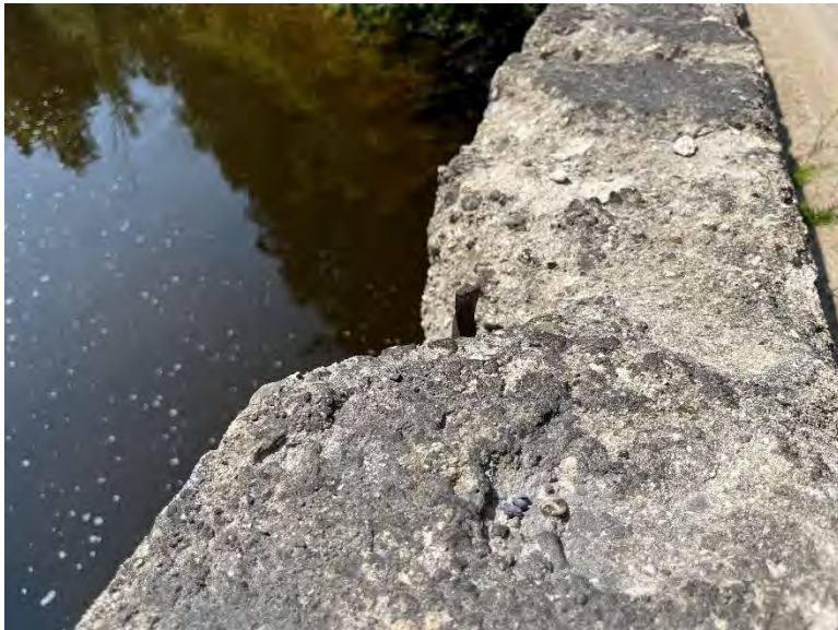
Figure 18: Detail view of exposed rebar on concrete barrier (A.S.I., 2023).
