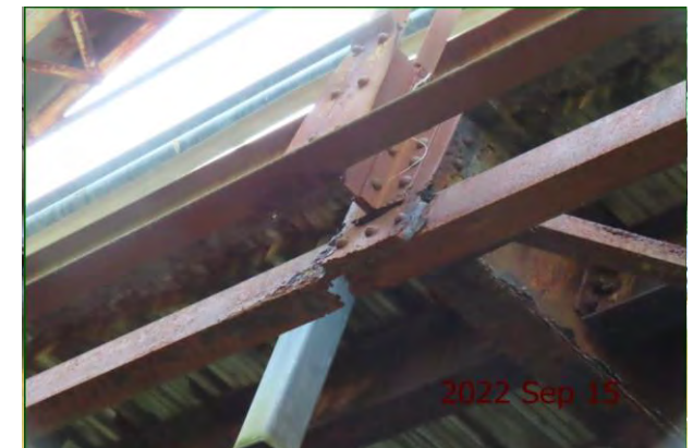
Severe corrosion and Severed Bottom Chord
