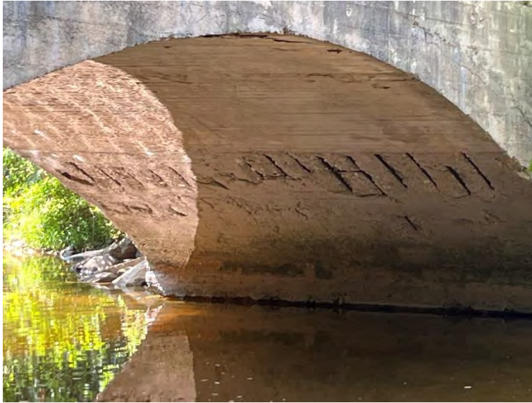
Figure 15: Detail view of barrel soffit showing concrete deterioration and exposed rebar (A.S.I., 2023).
