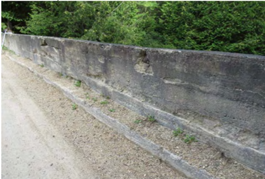
Figure 2.6 Deterioration of Parapet Wall
