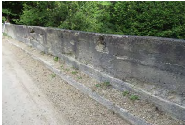
Deterioration of Parapet Wall
