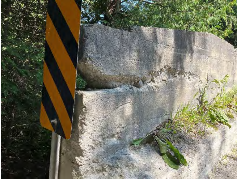
Figure 17: Detail view of significant deterioration on barrier and growth of vegetation on curbs on western approach (A.S.I., 2023).
