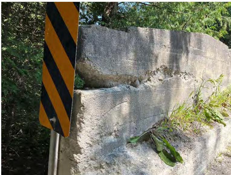
Plate 9: Detail view of significant deterioration on barrier and growth of vegetation on curbs on western approach (A.S.I., 2023).
