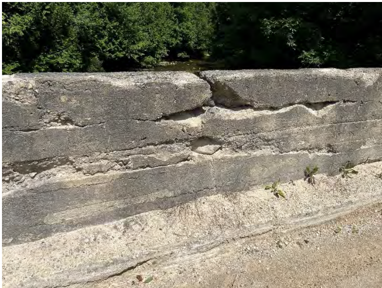
Plate 11: Detail view of significant deterioration to concrete barrier and curb (A.S.I., 2023).
