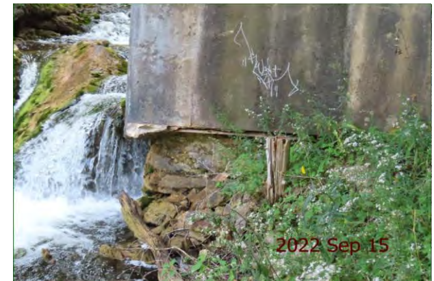
Partial Foundation Exposed and Disintegrated, Undermined.
