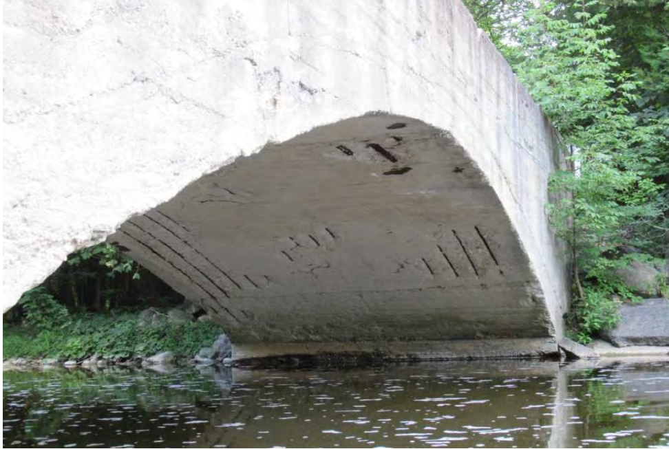
Figure 2.9 Exterior and Interior Soffit with Spalling and Exposed Rebar
