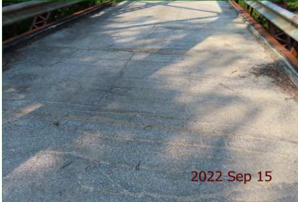
Medium to Wide Transverse Cracks Throughout Approach
