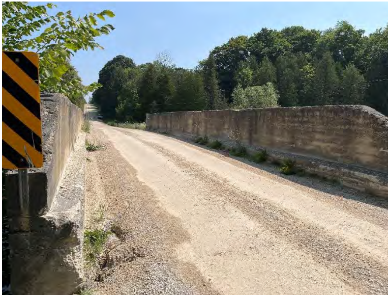
Figure 26: Detail view of the deck, barriers, and curbs of the North Line Saugeen River Bridge (A.S.I., 2023).
