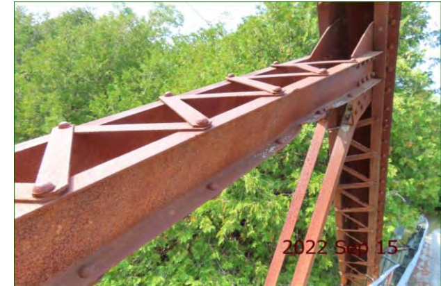
Impact Damage on Diagonals
