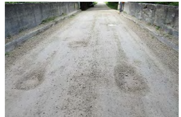
Potholes and Wheel Path Rutting on Structure Wearing Surface
