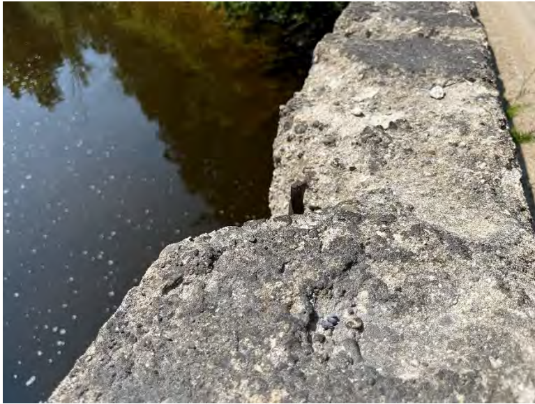
Plate 10: Detail view of exposed rebar on concrete barrier (A.S.I., 2023).
