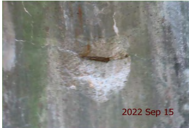
Severe Spall with Exposed Reinforcement
