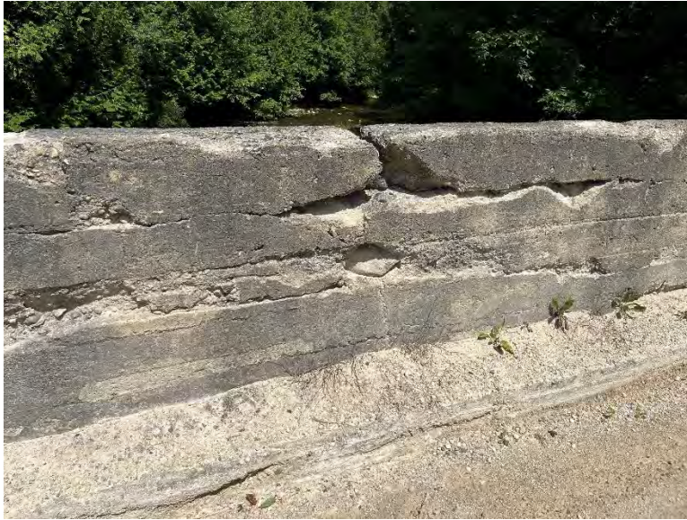
Figure 19: Detail view of significant deterioration to concrete barrier and curb (A.S.I., 2023).
