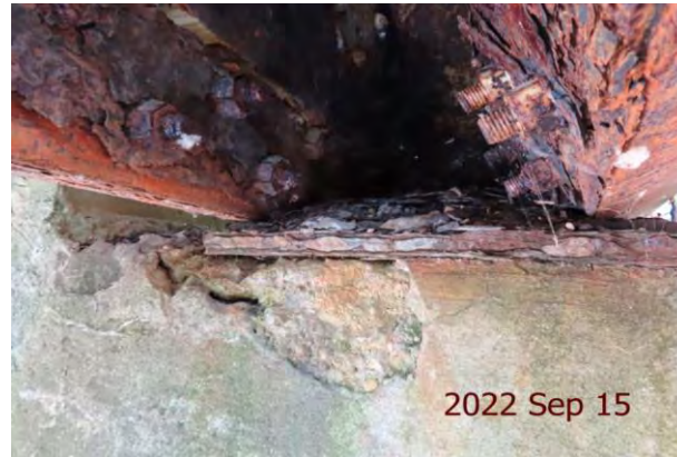
Medium to Severe Corrosion Throughout Bearings
