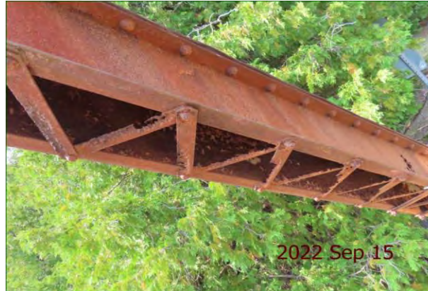
Severe Corrosion and 100% Section Loss
