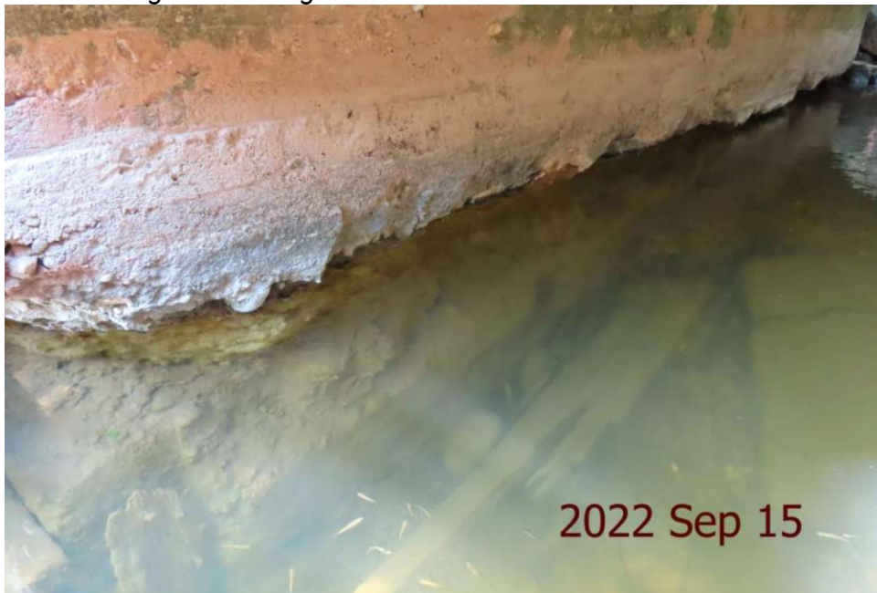
Figure 2.8 Severe Scouring and disintegration at Waterline
