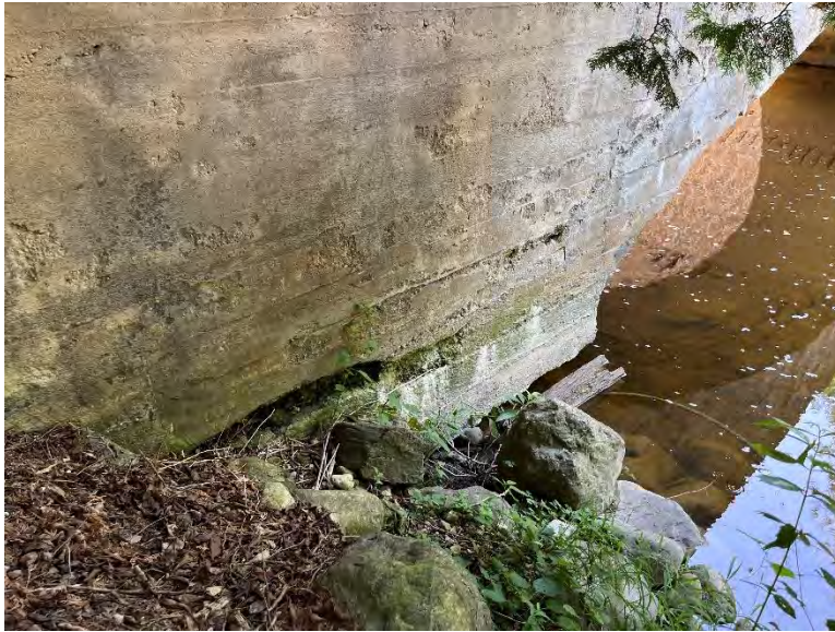
Plate 6: Detail view of north side of eastern abutment. Significant deterioration is visible at the waterline and at the berm (A.S.I., 2023).
