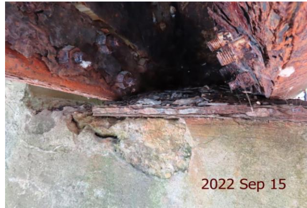
Medium to Severe Corrosion Throughout Bearings
