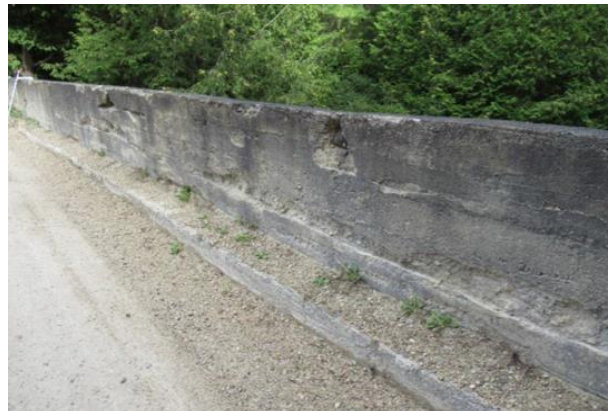
Deterioration of Parapet Wall
