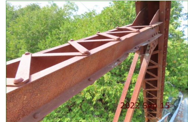
Impact Damage on Diagonals
