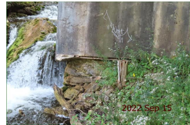
Partial Foundation Exposed and Disintegrated, Undermined.
