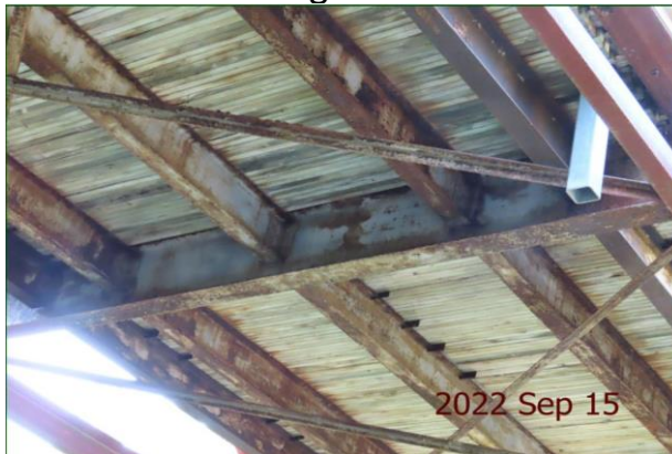
Severe Corrosion at Ends on Floor Beam
