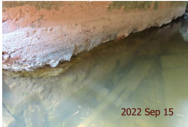
Barrel: Severe scouring and disintegration at waterline
