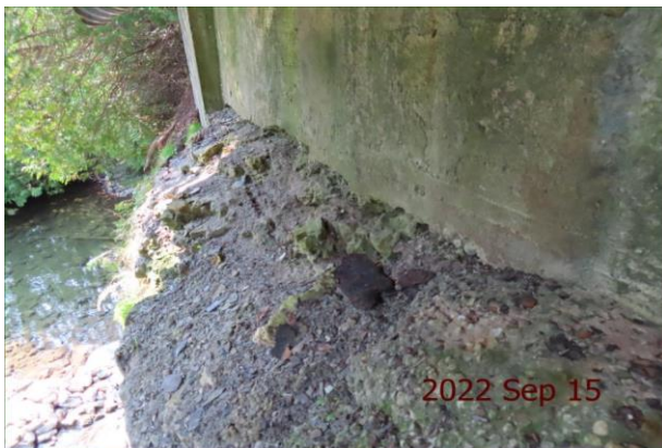
Severe Scouring and Disintegration Along Bottom of Abutment
