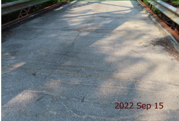
Medium to Wide Transverse Cracks Throughout Approach
