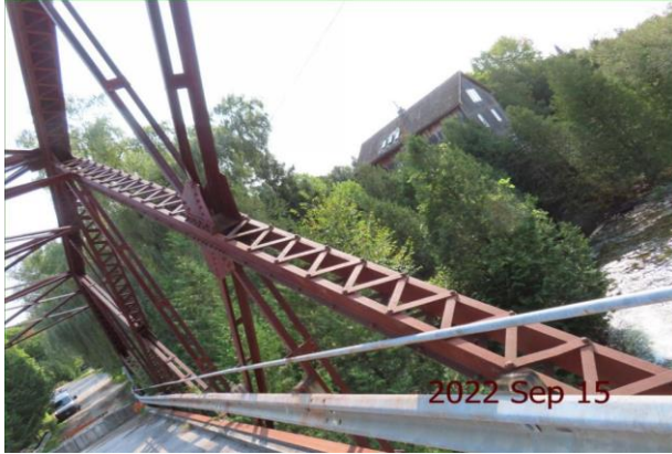
Corrosion and Impact Damage to Diagonals
