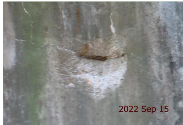
Severe Spall with Exposed Reinforcement
