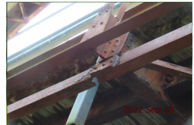
Severe corrosion and Severed Bottom Chord
