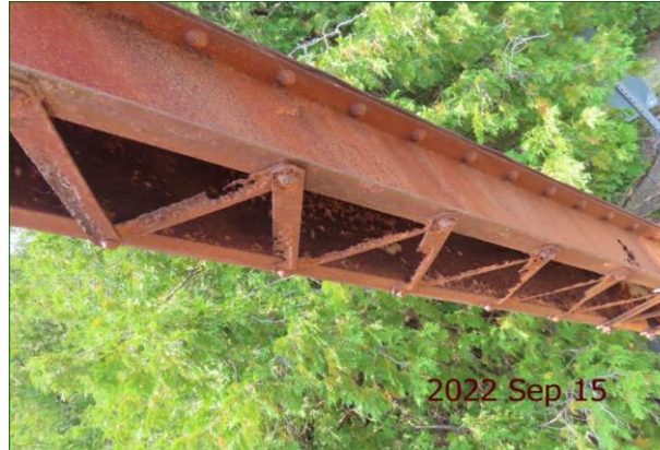
Severe Corrosion and 100% Section Loss
