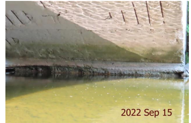
Barrel: Severe scouring and disintegration at waterline
