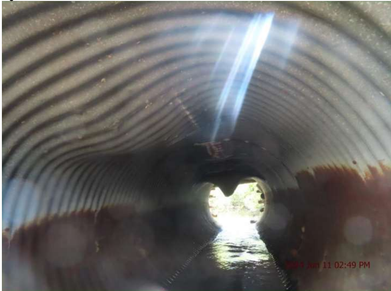
Figure 4.03: EG-001 Structure Failure
